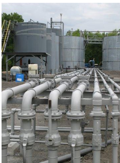
Tank Battery and Flow lines
